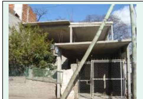
This butcher shop under construction was mostly funded by local individuals, who were also applying for some government funds in order to complete the project.
